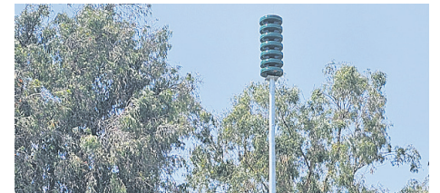
Photo courtesy city of Beverly Hills The city began installation of its Outdoor Warning Siren network.
