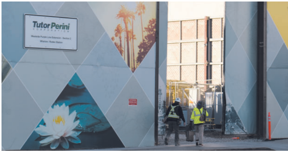
Workers walking into the construction site at the future LA Metro subway station at Wilshire Boulevard and Reeves Drive. Photo by Carl Robinette
