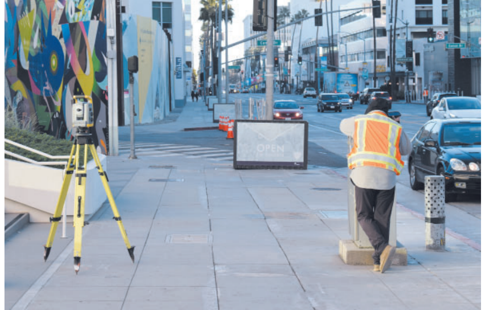
Surveyor checks his phone while working on the future LA Metro subway station at Wilshire Boulevard and Reeves Drive. Photo by Carl Robinette
