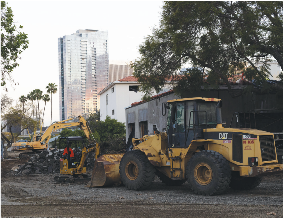
Ongoing construction at El Rodeo School under the school's bond program Photo by Samuel Braslow
